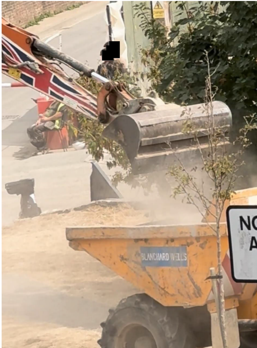
Photo 5 taken July 2026 showing the effect of the dust and utter lack of mitigations because of the absence of a CEMP. This dust will contain silica and cement particles, which causes permanent long term damage to lung health including COPD and other chronic health issues and allergies.
